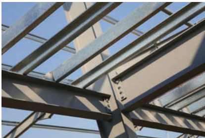
Beam-to-column connection with one beam attached to column flange and other attached to column web
