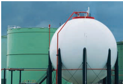
Thin-walled spherical pressure vessel used for storage of propane in this oil refinery
