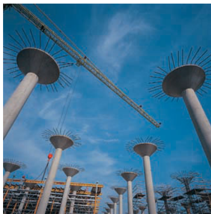
Slender concrete columns fixed at the base and free at the top during construction
