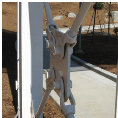
Diagonal bracing for an elevated walkway showing a clevis and a pin in double shear
