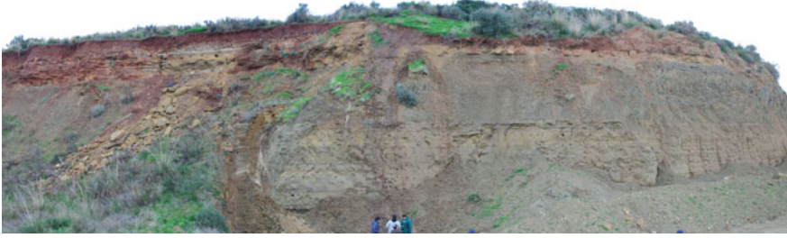
Fig. 2.101 Stratigraphic relationships—marked by subaerial erosional unconformity—between the clayey sands of the marine terraces of the Buonformello synthem and the overlying continental deposits (colluvium and red soils) of the Capo Plaia synthem (Contrada Pestavecchia, Buonformello, Termini Imerese Mountains)
