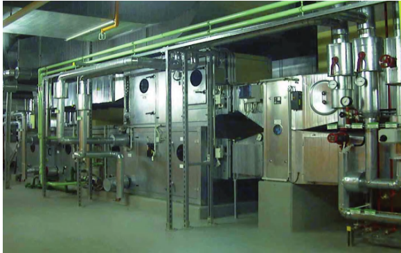
Fig. 3-49 Conventional climate control room
