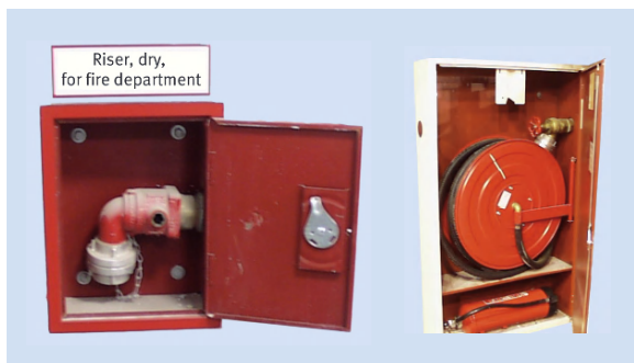
Fig. 3–34 Point of withdrawal for firefighting water and wall hydrant
