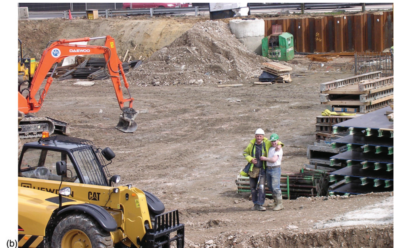
Figure 19.3 (a) Poor conditions – inspection needed; (b) passed inspection?
