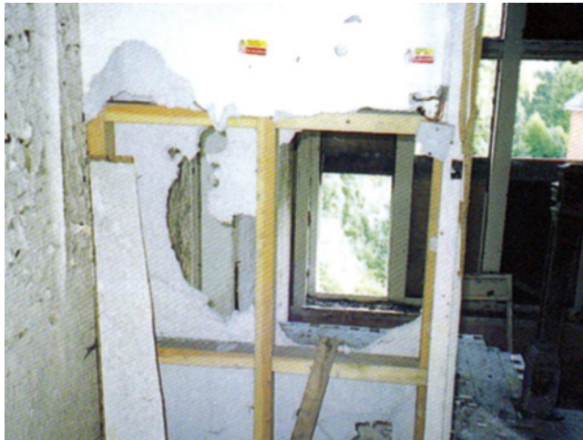
Figure 16.15 AIB wall panels badly damaged during poorly planned and uncontrolled work.
