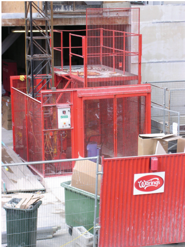
Figure 8.11 Hoist with interlocked gates.
