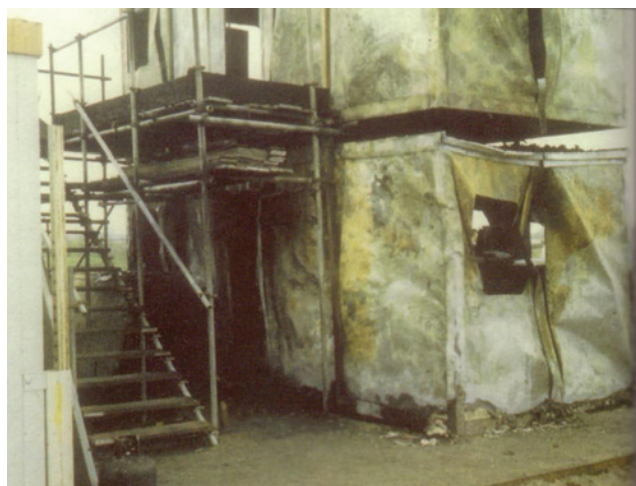
Figure 15.9 In this fire, leaking gas ignited and a man died despite the escape stairway.
