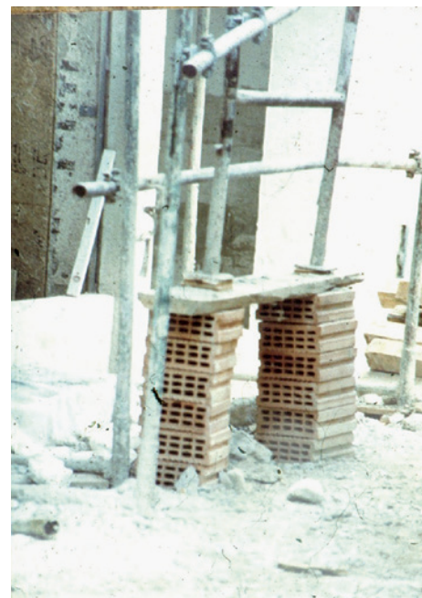
Figure 18.2 Unsafe scaffold – accident waiting to happen.
