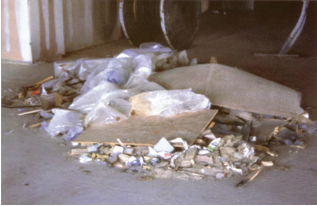
Figure 4.4 Most construction rubbish can burn. Make sure that it is swept up and removed from the site as soon as possible.
