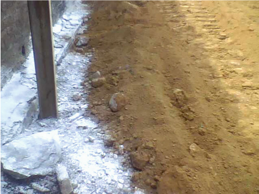
Fig. 3 Fire combated portion treated with binding material with top soil near mining workshop and Giddi power substation, CCL
