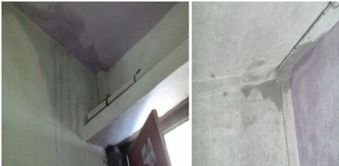
Fig. 10 Seepage of water from joint of beam and brickwork. Source Authors
