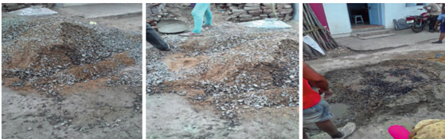
Fig. 6 Aggregates are mixed with improper graded stones and last picture shows poor mixing of concrete. Source Authors
