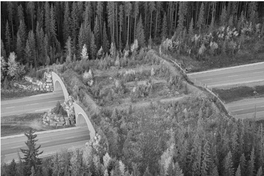
Figure 1.2. One of the Bow Valley Wildlife overpasses across Highway 1, part of the Banff Wildlife Crossings Project in Banff National Park, Alberta. (Photo by Steve Michel, Banff National Park.)
