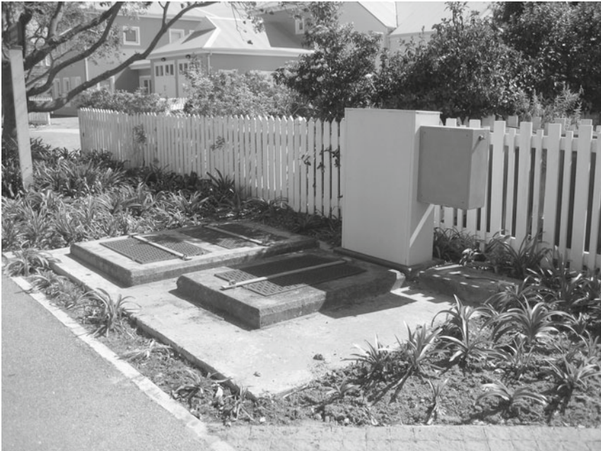
Figure 5-3. An example of utilities integrated harmoniously into the design of the street in a residential subdivision, designed by Chris Mulder Associates Inc. (Source: Michael Murphy.)
