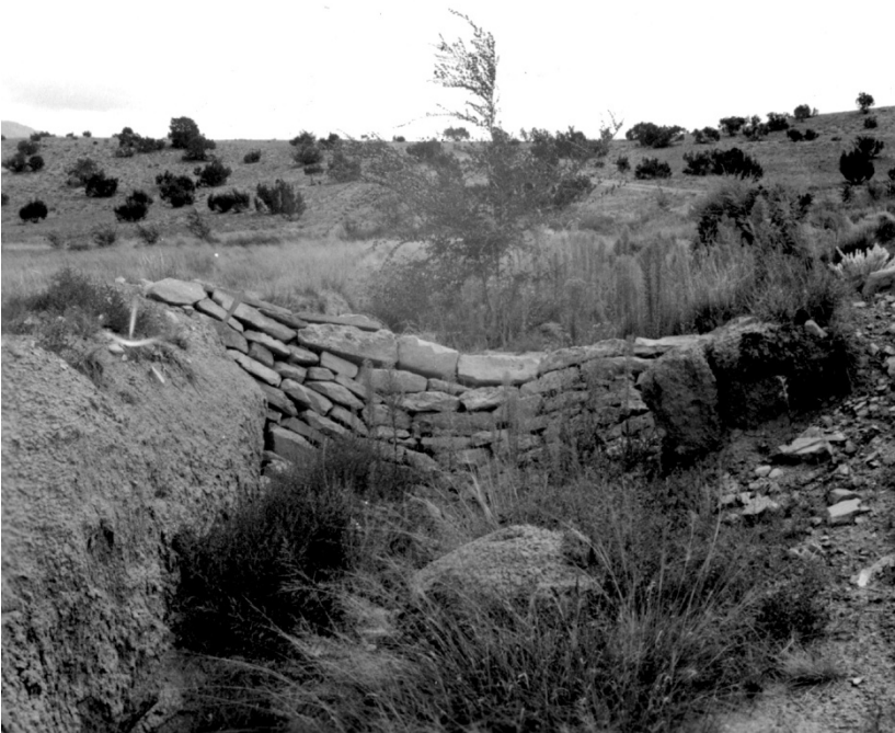
Leopold returned to the Southwest for a few months in 1933 to oversee government erosion control work, including the construction of check dams—structures built to plug gullies and prevent their spread. In this photograph, taken in New Mexico a few years later, a gully is showing signs of healing, supporting a good growth of grass.
