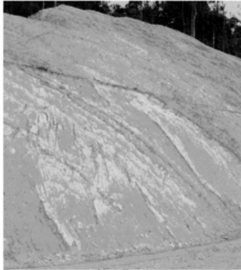
Figure 5.34. Joints with infilling material.
