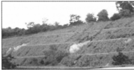
Figure 7.6. Localised slip failures and erosions on slopes.
