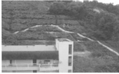
Figure 5.54. Front view of failed slope.
