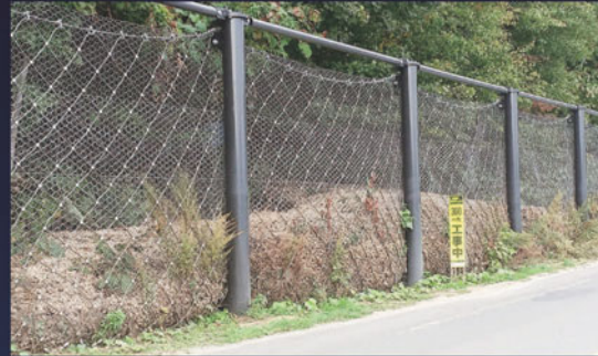
SLOPE GUARD FENCE: Slope failure protection fence caught soil of slope failure caused by a heavy rain.
