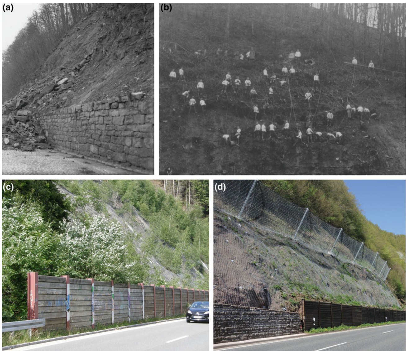
Fig. 3 Development of mitigation measures in southern Lower Saxony, NW Germany. a Rockslide event (02/1937) in the Upper Weser area. The drywall in the front stabilizes slope with no protection against rockfalls/slides. b Removal of loose rock and vegetation in the Upper Weser area in 1936. c Combination of steel buttress/wooden
