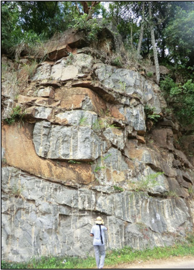
Fig. 5 This relatively old cut slope indicates progressive erosion, with unsupported or over-steepened slope conditions and degradation over time. The detachment of larger blocks or volumes of falling rock produces greater impact forces than smaller events. This type of rockfall is commonly caused by erosion that leads to a loss of support, either locally or throughout the slope
