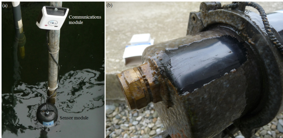
Fig. 13. (a) Second generation phosphate analyser in-situ at Osberstown Wastewater Treatment Plant, Co. Kildare, Ireland. (b) Biofouling on the analyser body after approx. 2 weeks immersion in wastewater.
