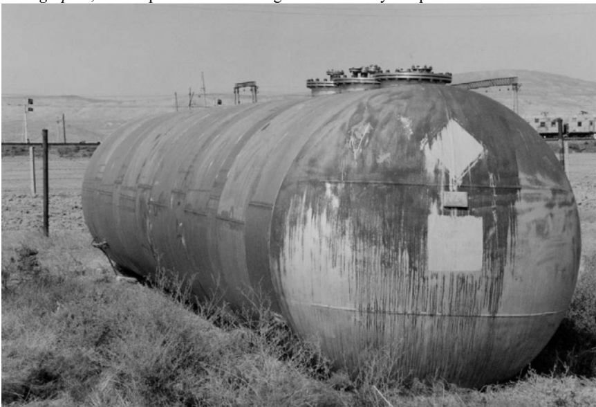
Photograph 6 , Close-up of a Samine storage tank at the Alyat depot.
