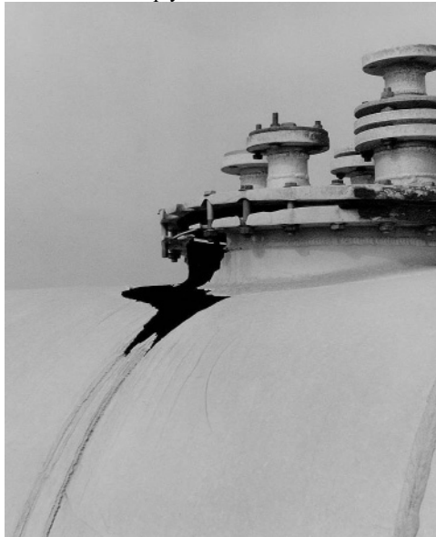
Photograph 8 , Close-up of a large leak at the top/cap of an oxidizer storage tank at the Mingechevir depot. The tank is now empty.
