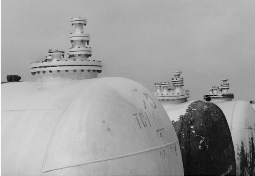
Photograph 7 , Close-up of oxidizer storage tank caps at the Mingechevir depot. As in Alyat, safety valves have corroded away and are lying on the ground. Nitrous gases escape continuously.
