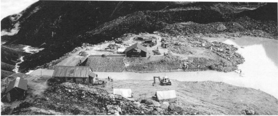
Figure 3: The nearly completed spillway at Tsho Rolpa (4,500 m), Rolwaling Himal, Nepal, in 2000. The lake level was lowered successfully by 3.5 m following construction of the new spillway and sluice gates. It took from April 1999 to July 2000 to complete the works at a cost of ca $3 million. Heavy machinery had to be flown to the site in bits and reconstructed at site. Glacier ice is still present within the moraine dam (right-hand side of picture). Although the glacial hazard has been reduced significantly, it has been recommended that the lake level should be drawn down at least a further 11.5 m to ensure an adequate factor of safety for the 150-m high moraine dam (Photograph © Reynolds Geo-Sciences Ltd, 2000).
