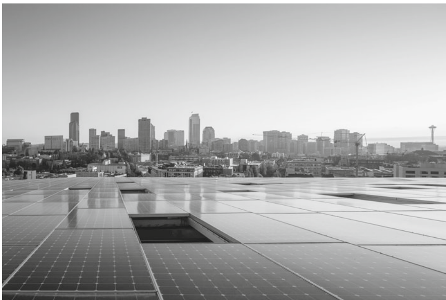
Figure 3-10: Near-Flat Solar Array at the Bullitt Center
