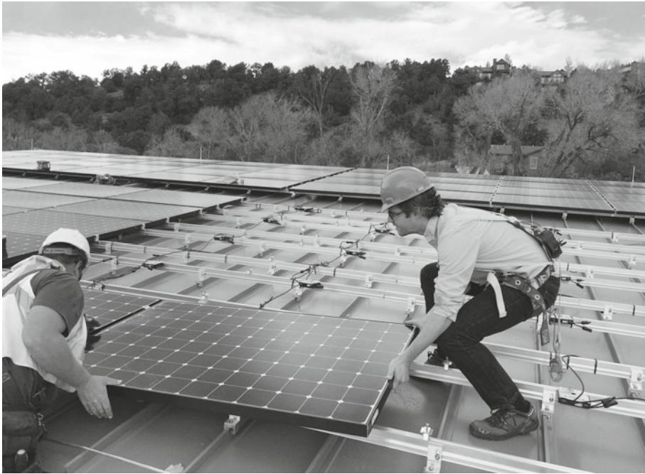
Figure 3-3: Typical Solar Panels
