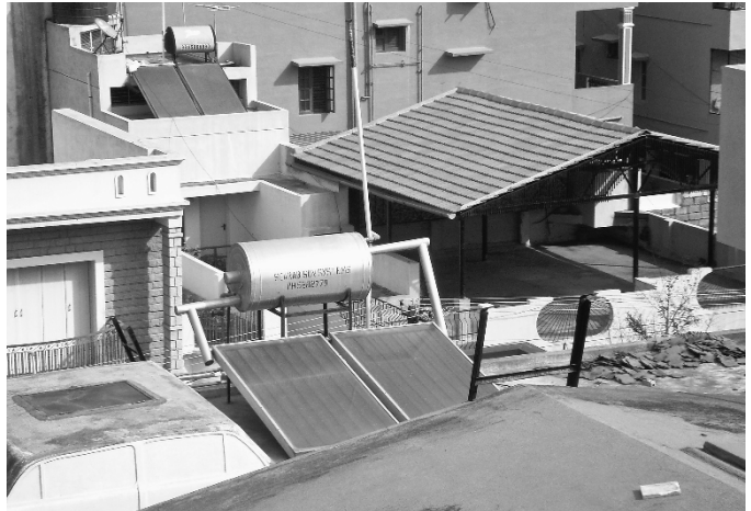
Solar water heaters in Bangalore, India.
