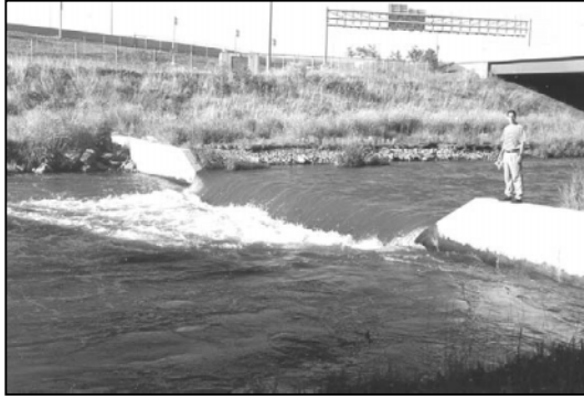
Figure 10. A 0.8-metre high “killer drop” in Clear Creek; a site of two drownings. “Keeper” at the downstream face has currents that pull objects against the drop. Photograph by permission of Wright Water Engineers, Inc.
