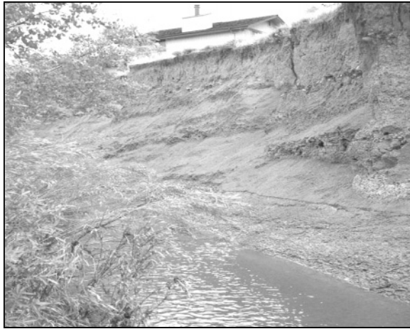
Figure 2. Willow Creek's eroded bank threatens homes. Photographs by permission of Urban Drainage and Flood Control District
