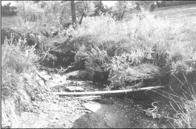
Figure 5. Degraded Goldsmith Gulch through Bible Park, note exposed utility line. Photograph by permission of Urban Drainage and Flood Control District
