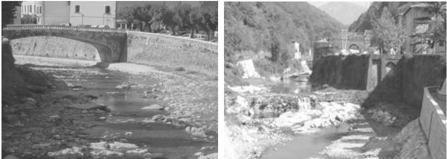
Figure 1. Sill grade control (left) and wall with concrete toe protection (right) in a mountain urban stream
