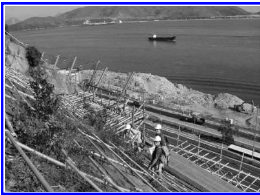
Figure 14. Steep rock slope to be excavated to accommodate widened expressway in Hong Kong (Pine & Roberds 2005).
