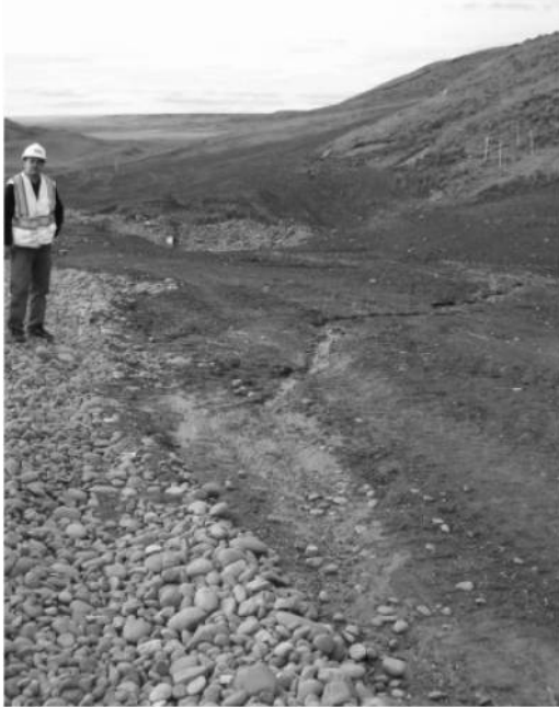
HPIM0371 2004-09-20 Missing armoured section at culvert inlet, erosion has started.
