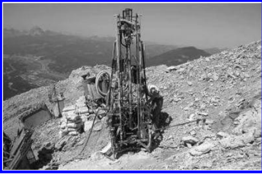
Figure 9. Air rotary drill used on South Peak during installation of subsurface geophones.
