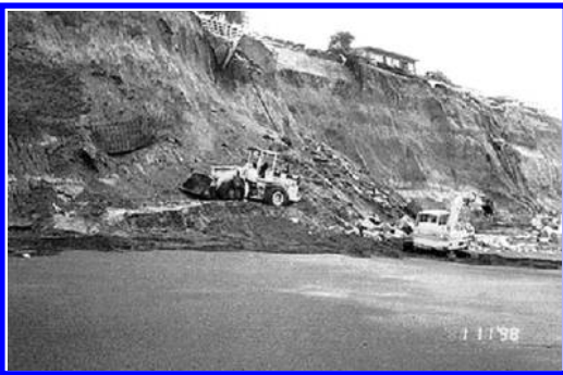
Figure 2. Removal of homes in Pacifica, California, USA following 1998 bluff failures (USGS photo).
