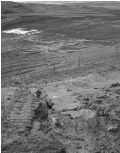
HPIM0377 2004-09-20 Erosion problem on west embankment face of the fill section.
