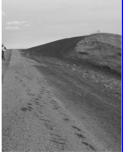
HPIM0372 2004-09-20 West ditch at grade point, no armoured ditch, erosion has started.
