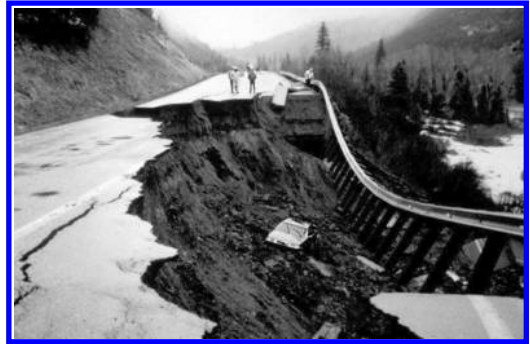
Figure 5. Loss of service due to landslide at McClure Pass Colorado (note car on landslide) (by USGS).
