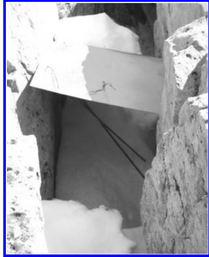
Figure 10. Vibrating wire crackmeters installed across a major fissure. The metal snow roof is to protect the instruments.
