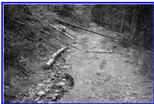
Figure 11. Evidence of redirected water down the forest road.
