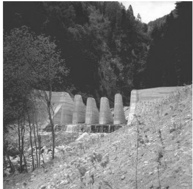
Figure 5 Slit check dam with a series of debris-flow breaker on Torrent Chieppena – Trentino Italy (Provincia Autonoma di Trento, 2002). A color version of this image is available at http://www.mrw.interscience.wiley.com/ehs
