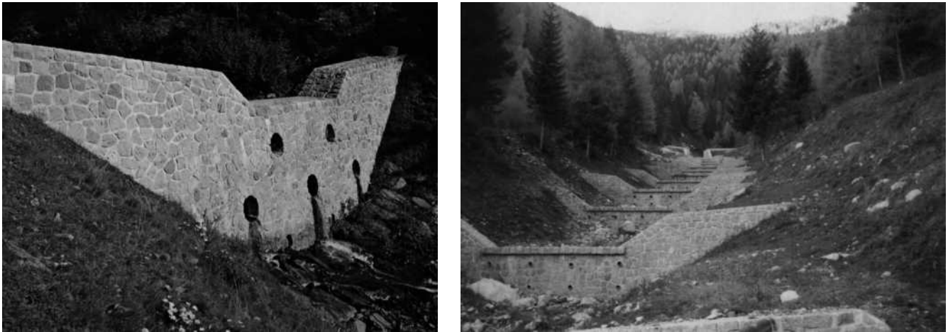
Figure 6 Retention check dam (Provincia Autonoma di Bolzano Alto Adige, 1977) (a) and sequence of consolidation check dams Rio Val de Casa (b) (Provincia Autonoma di Trento, 1991). A color version of this image is available at http://www.mrw.interscience.wiley.com/ehs
