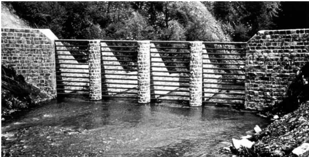
Figure 7 Beam dam in Tyrol, Austria. A color version of this image is available at http://www.mrw.interscience.wiley.com/ehs
