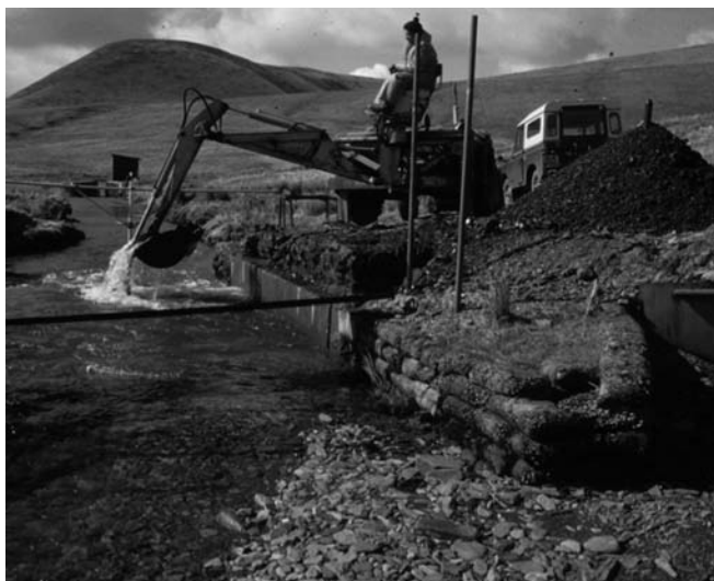
Figure 3 Emptying of a bed-load trap at the CEH upland experimental catchments, Plynlimon, Mid Wales, UK. A color version of this image is available at http://www.mrw.interscience.wiley.com/ehs
