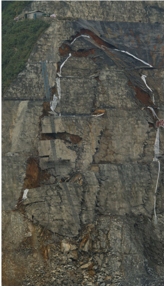
Fig. 9.27 Right abutment slope after the local collapse
