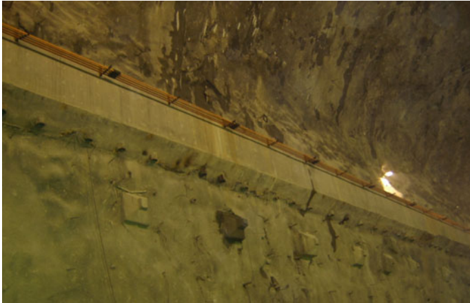
Fig. 15.58 Details showing the rock bolt crane girder (left wall): Saizhu Project, China
