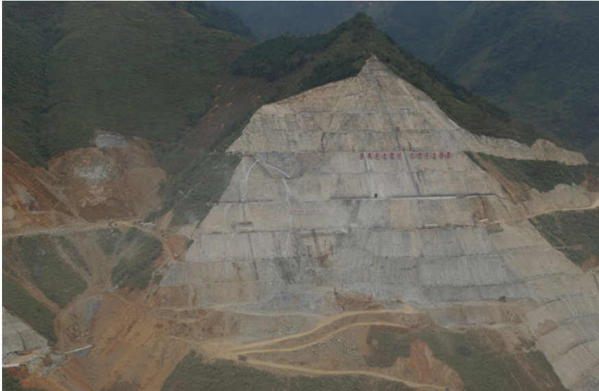
Fig. 9.26 Right abutment slope before the local collapse
