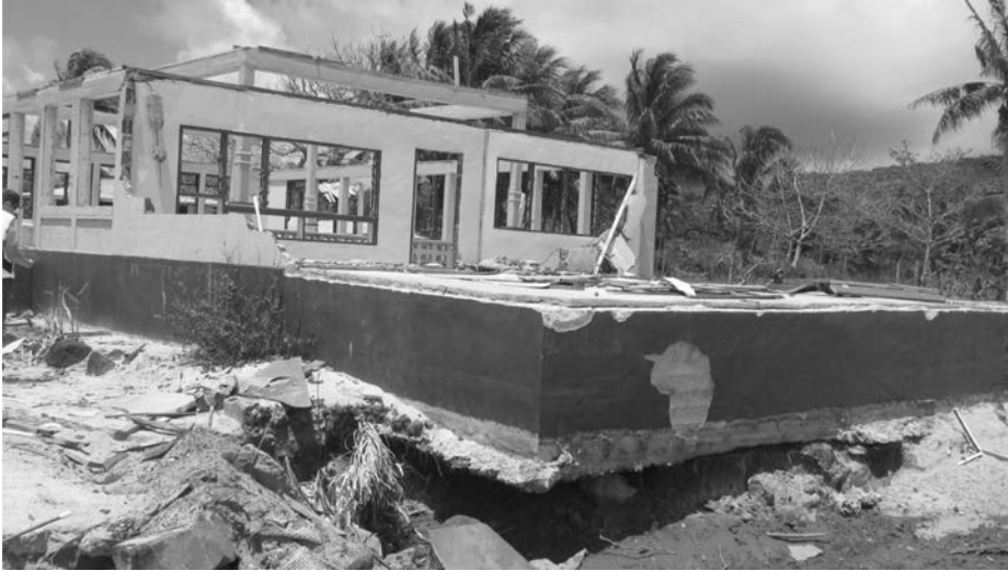
Figure 4.27 An example of the damage to buildings caused by the tsunami on Samoa. Note the undermining of the foundation due to scour as well as the damage to roof and walls. (Photograph courtesy of Dr. Alison Raby.)
