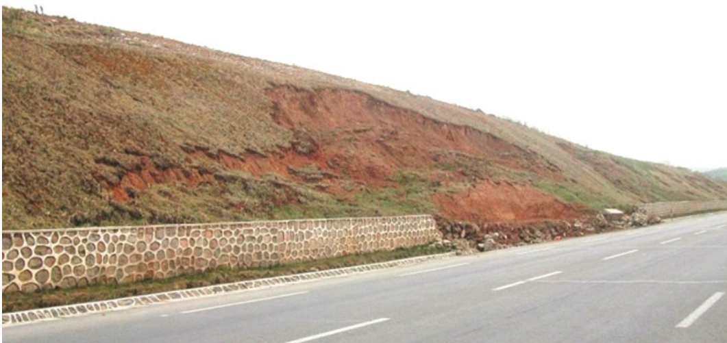
Fig. 1 Typical failure of cutting slope
