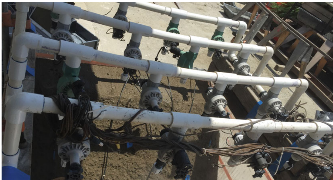
Fig. 4 Example of rain simulator system consisting of 16 sprinkler heads with adjustable nozzles connected with PVC piping to the desired spacing
