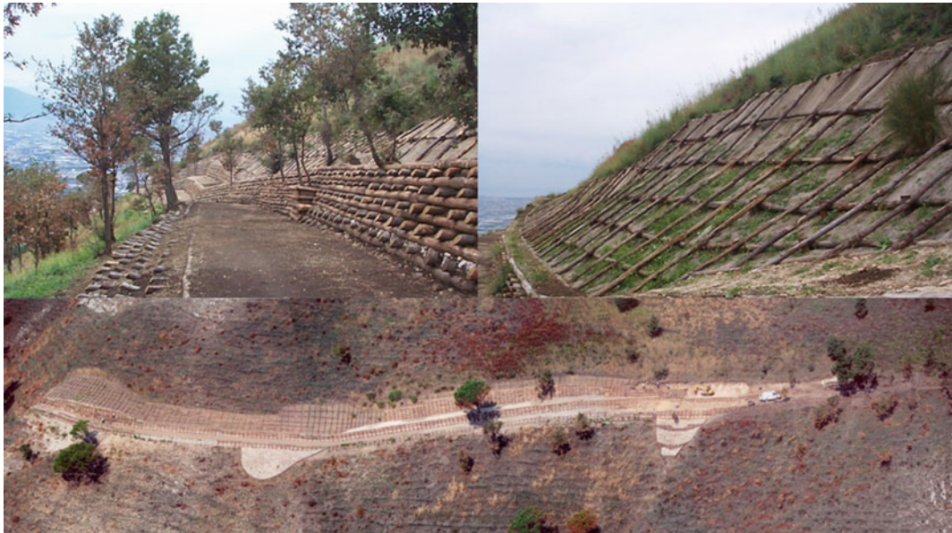
Fig. 4 Example of bioengineering works along Pizzo d'Alvano side. Down in particular, a top view of the work during the construction phase
