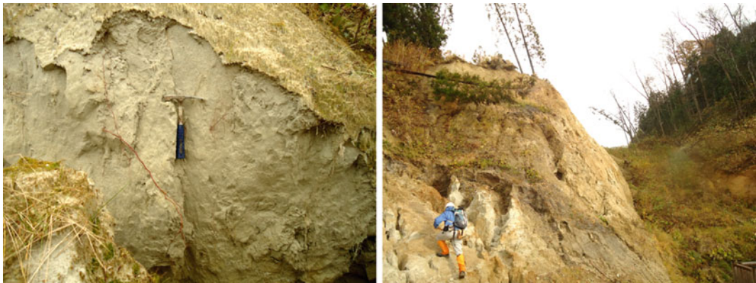
Fig. 3 Observing landslide debris material within block ( top ) and at the toe part ( bottom )
