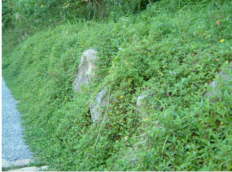
Fig. 8 Vegetation invasion on revetment
