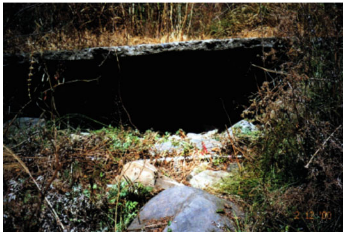
(c) Soil erosion
