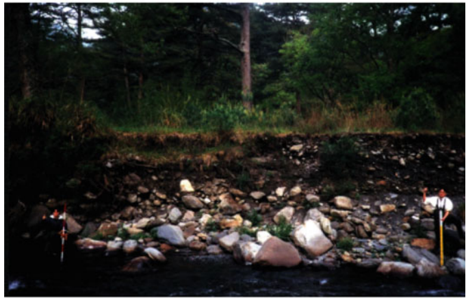
(b) Riverbank landslide
