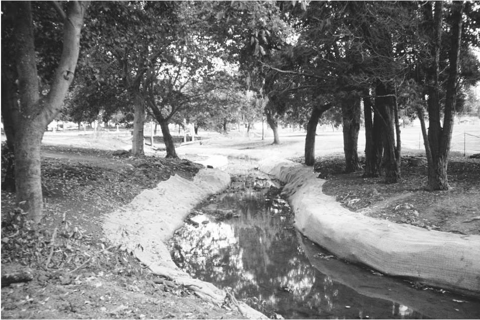
FIGURE 3.49 Baxter Creek at Anderson Park was regraded to equilibrium dimensions and meandered under existing large trees, as shown here in 2000. Photo credit: Lisa Owens Viani.
