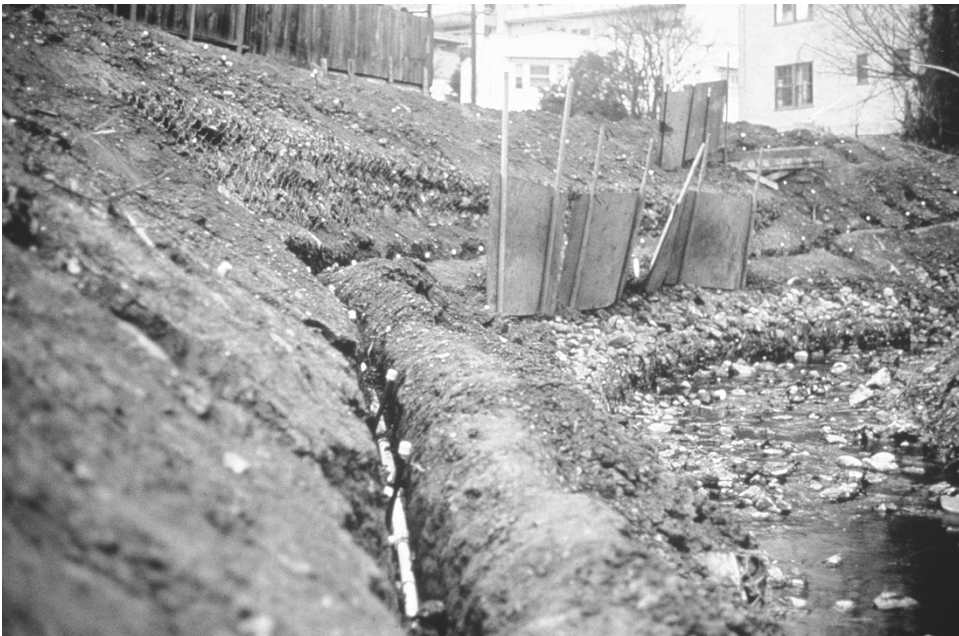
FIGURE 3.10 Glen Echo Creek was reconstructed using gabions filled with dirt and an irrigation system to support revegetation.
