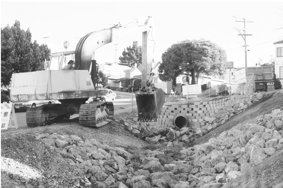
FIGURE 3.37 The concept design guiding the design-build step pools employed a range of sizes of boulders and cobbles. Most of the rock in this photo was removed.
