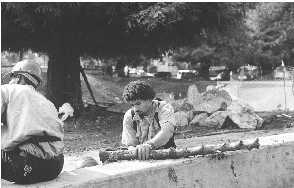
FIGURE 3.23 Posts, sometimes called poles, are cut and prepared from willow plants and are larger than stakes. Posts are installed in high shear stress areas. They can range from 3 to 10 feet long and 3 to 5 inches in diameter.
