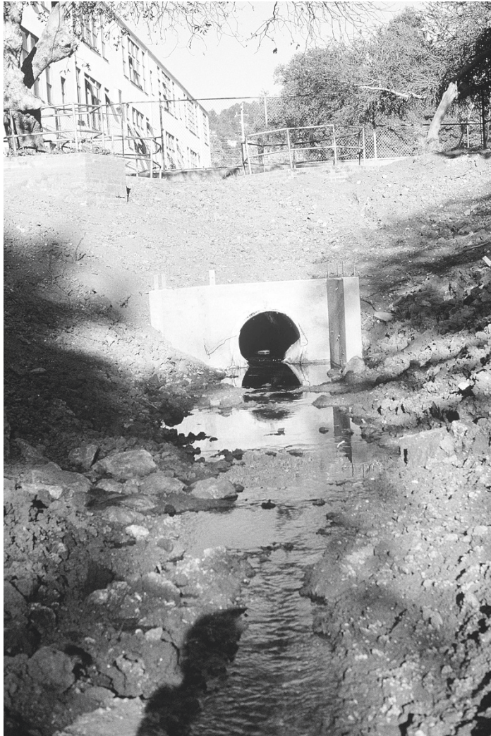
FIGURE 3.20 New headwalls were constructed around both the upstream and downstream ends of the Blackberry Creek cut culverts.
