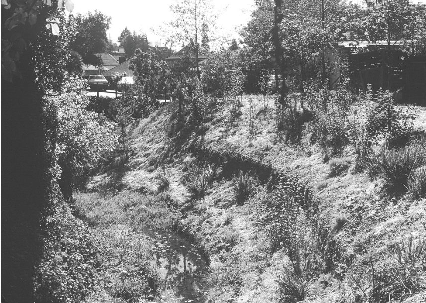
FIGURE 3.13 The reconstructed Glen Echo Creek channel was planted with a range of native riparian plants, including ferns, shrubs, and trees. This photo was taken in 1988, three years after installation.
