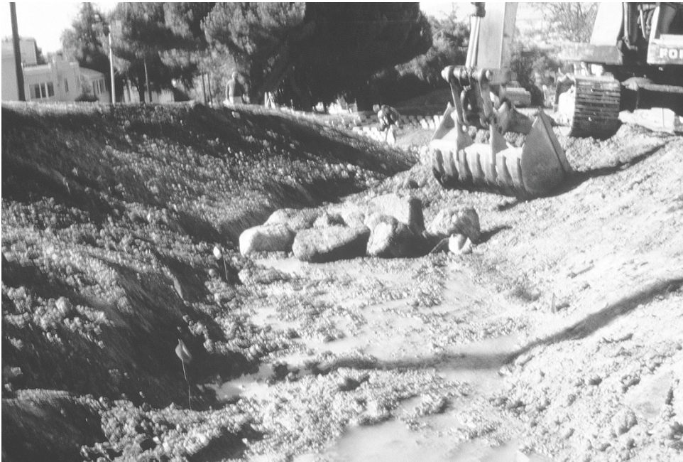
FIGURE 3.38 Some rock was salvaged from the first engineering project on the channel to build the step pool channel at Baxter Creek.
