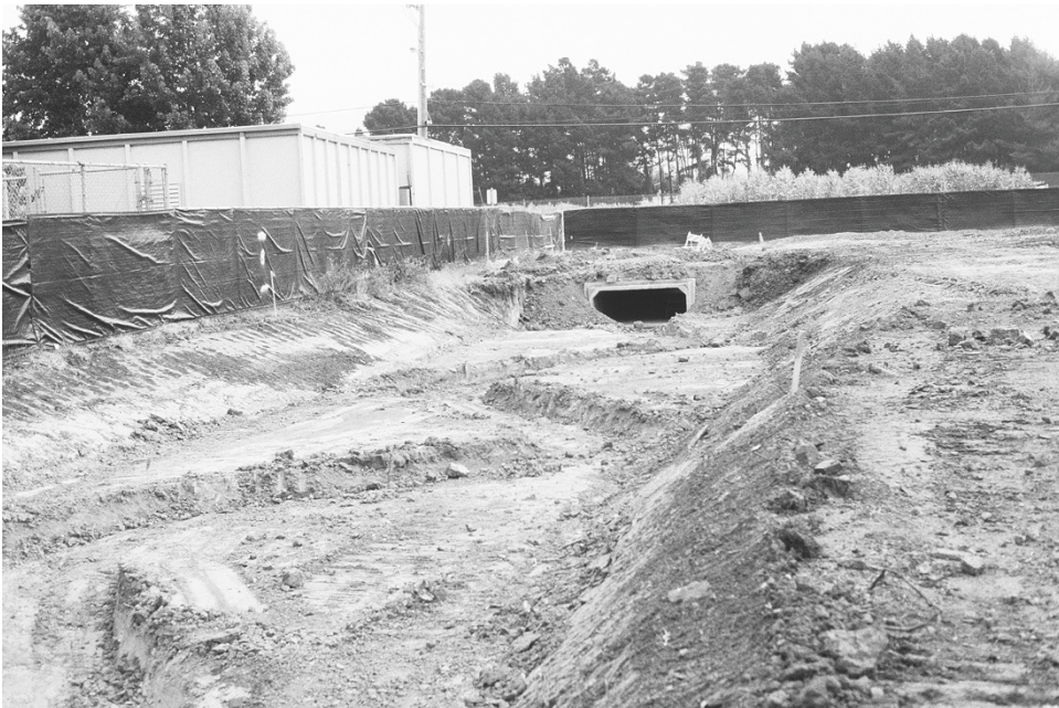
FIGURE 3.61 An active channel and floodplain were excavated in Village Creek's trapezoidal corridor.
