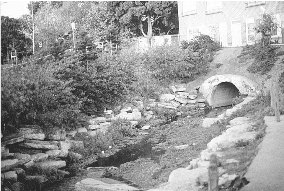
FIGURE 3.5 The Strawberry Creek construction project was completed in 1983, keeping most demolition materials on the site. Photo credit: Gary Mason of Wolfe Mason Associates.
