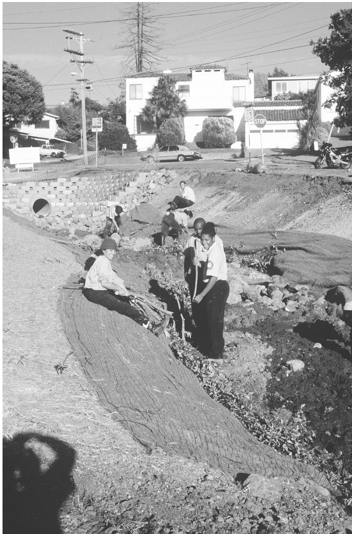
FIGURE 3.39 The East Bay Conservation Corps completed the final grading, fabric installation, and soil bioengineering for the Baxter Creek project.
