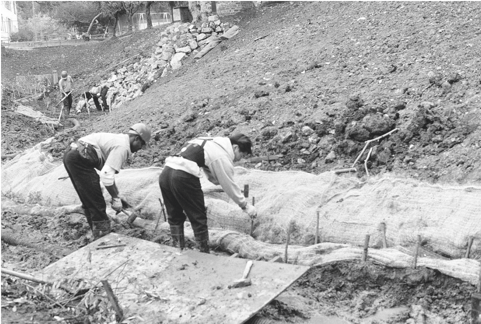
FIGURE 3.21 Erosion control fabric was installed and fascines were added to secure the toe of slope.
