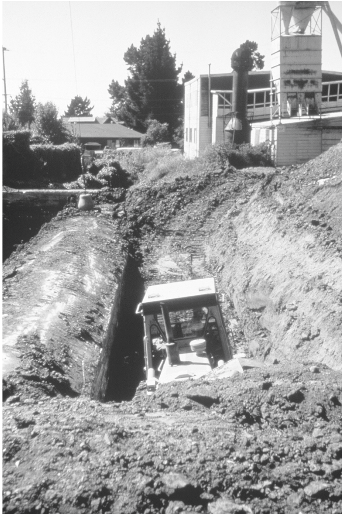
FIGURE 3.4 Both a wrecking ball and a front-end loader were needed to excavate the 1906 culvert at the Strawberry Creek site. Photo credit: Gary Mason of Wolfe Mason Associates.
