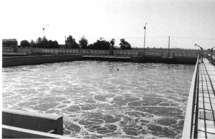
Figure 2. The activation tank of wastewater treatment plant II.
