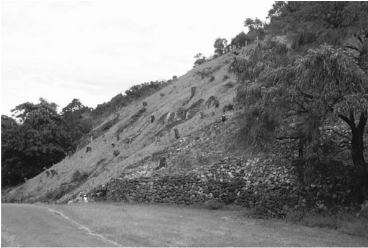
Fig. 16.2 Slope and Lower Walkway at Kings Park (©Survey Review: Gordon and Lichti [196])
