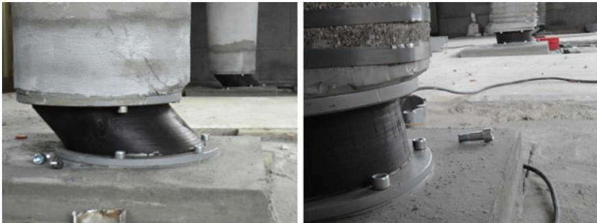
Fig. 15 Two of the elastomeric isolators in the deformed position, before returning to the vertical position. Left starting position. Right nearly final position
