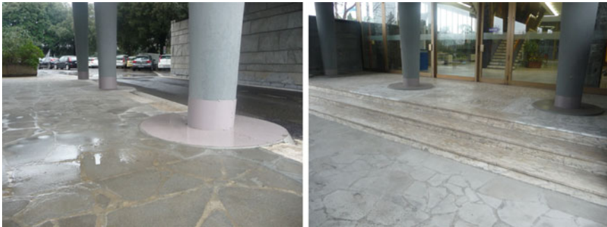
Fig. 17 Final phase of the work. The isolator devices are covered by metal protection cases. Left columns close to the driveway. Right columns at the lateral entrance of main hall
