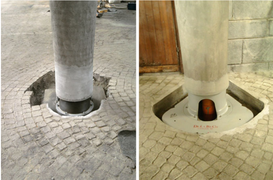
Fig. 16 Final position of elastomeric isolators
