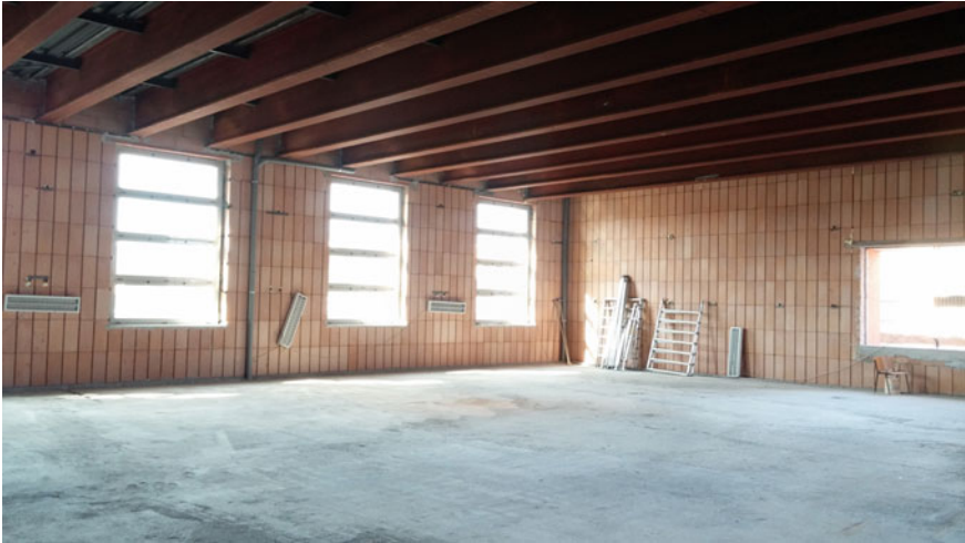
Fig. 9 A completed infill wall of almost 6 m in height, with and without openings
