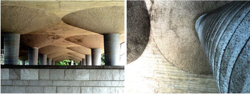
Fig. 9 View of the columns after shear strengthening with CAM system. Left west wing from main hall. Right bottom view
