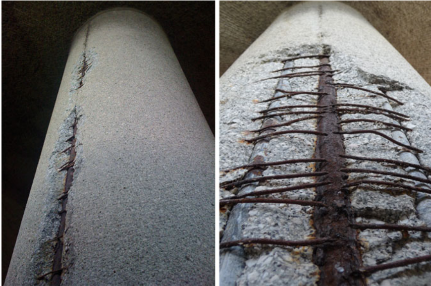
Fig. 8 Left mushroom-shaped column damaged by corrosion of bars. Right detail of the corroded longitudinal bars and transverse ties
