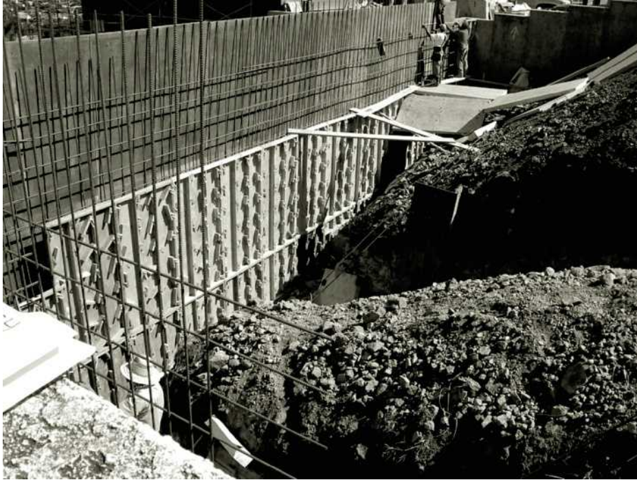
Figure 13.34 A cantilever retaining wall under construction (Courtesy of Dharma Shakya, Geotechnical Solutions, Inc., Irvine, California)
