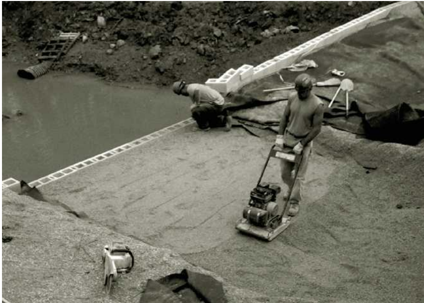
Figure 13.37 Construction of a retaining wall with geotextile reinforcement (Courtesy of Jonathan T. H. Wu, University of Colorado at Denver, Denver, Colorado)
