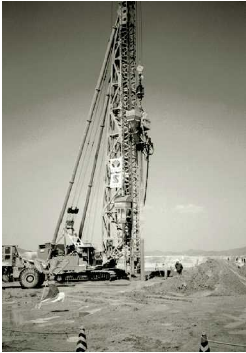
Figure 11.42 Sand drain installation in progress (Courtesy of E.C. Shin, University of Incheon, South Korea)
