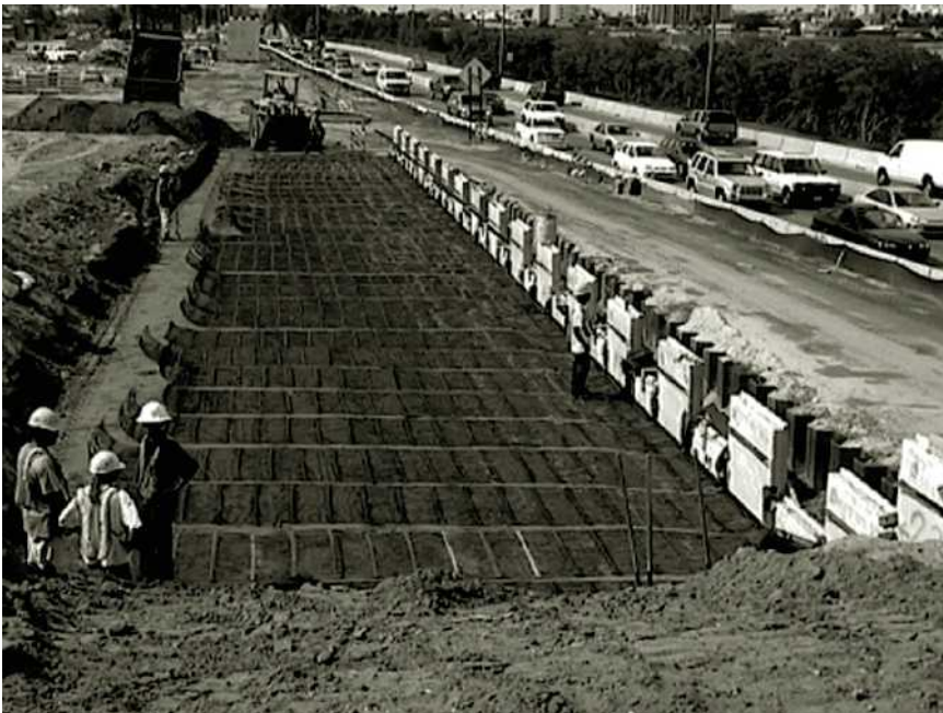
Figure 13.38 HDPE (high density polyethylene) geogrid-reinforced wall with precast concrete panel facing under construction (Courtesy of Tensar International Corporation, Atlanta, Georgia)
