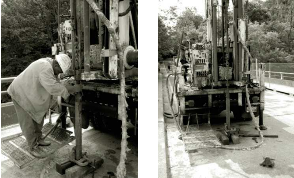
Figure 17.7 Drilling rod with split-spoon sampler lowered to the bottom of the borehole (Courtesy of Braja M. Das, Henderson, Nevada)
