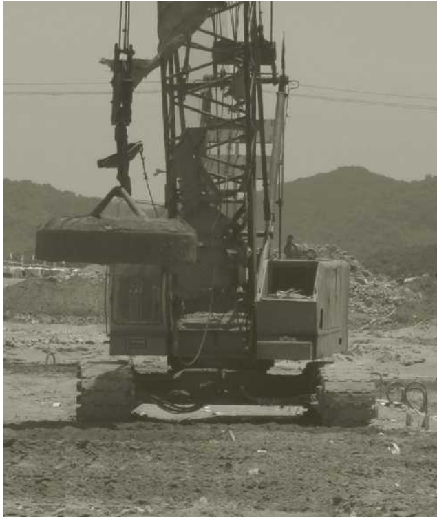
Figure 6.35 Dynamic compaction in progress (Courtesy of Khaled Sobhan, Florida Atlantic University, Boca Raton, Florida)
