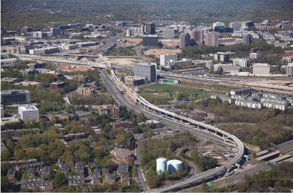
Figure 6.7. The Silver Line under construction in Tysons. This first phase, now open, has spurred millions of square feet of development around four stations in Tysons and one in Reston. (Virginia Department of Transportation, by Trevor Wrayton, under CC-BY NC ND 2.0)
