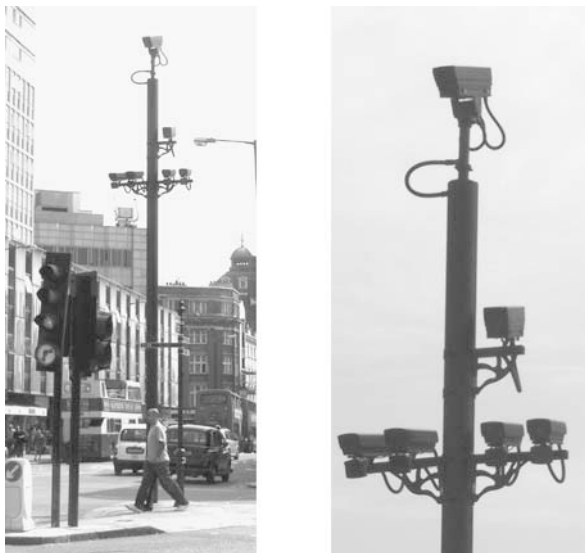
Figure 8.3 A typical camera installation
