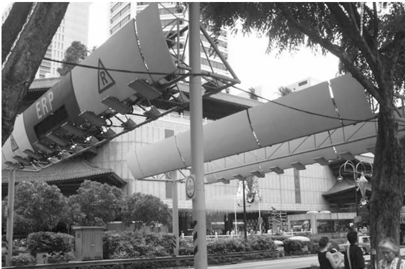
Figure 3.1 Singapore ERP: a typical roadside installation
