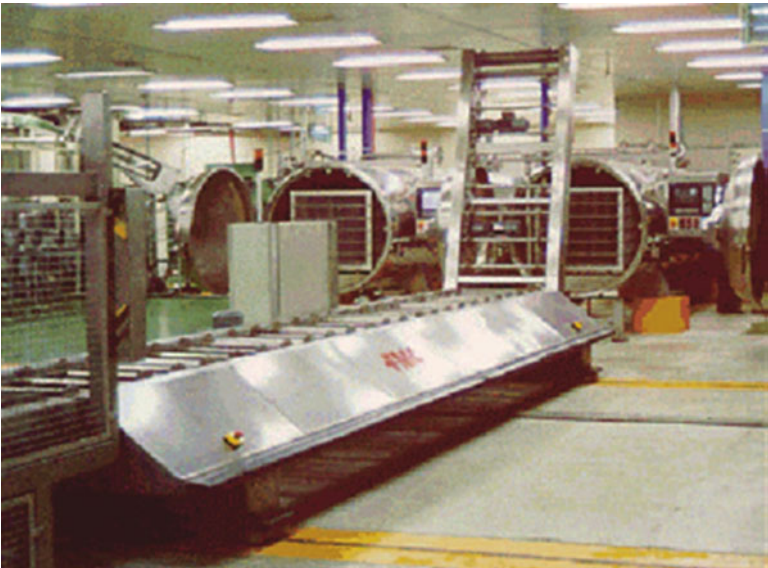
Fig. 21.8 FMC shuttle system for automated batch retort loading/unloading (Courtesy, FMC Food Tech., Madera, CA)
