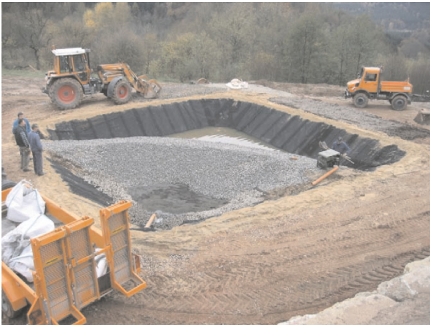
Figure 8. After excavation of soil and make the profile placement of the folia.
