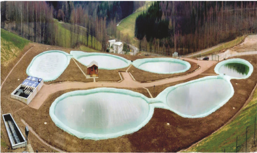
Figure 9. Aerial view of the full scale wetland at the Pöhla site. The double-line structure can be clearly seen, with one line in the upper part of the photograph and the second line in the lower. In the left lower corner, the aeration cascade is visible, followed by the rectangular settlement pond (concrete structure).
