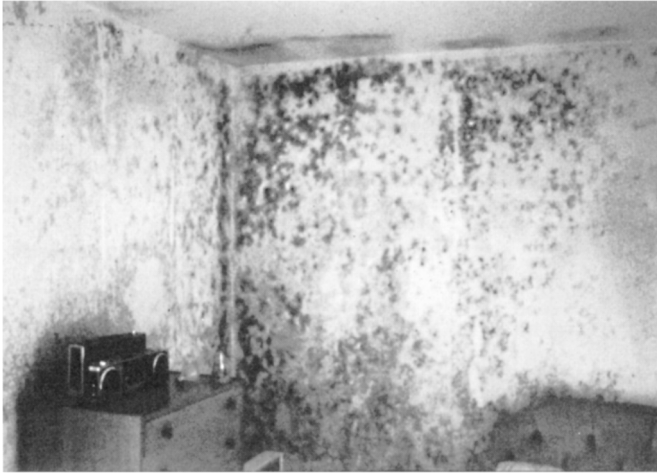
Figure 4.4 Mould growth on damp bedroom walls.
