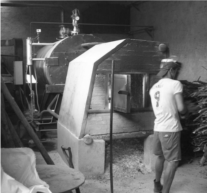
Fig. 9.2. Old steam boiler and furnace (source: photo taken by the author)
