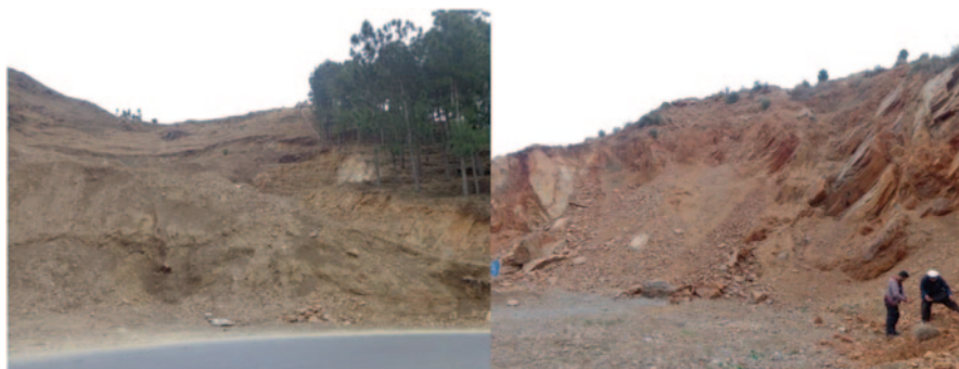
Fig. 14.16 Clearing a forest for construction of a hotel/resort for the visitors on Silk Road (Mansehra, KPK) on left. The thick forest trees are visible on the right side of the picture. Site cleared for shops on the roadside on Silk Road in Mansehra ( right )
