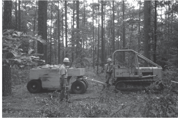
Fig. 23.5 Tractor-drawn Wobble Wheel used in our first soil compaction effort. Note ballast for adjusting the Wobble Wheel load
