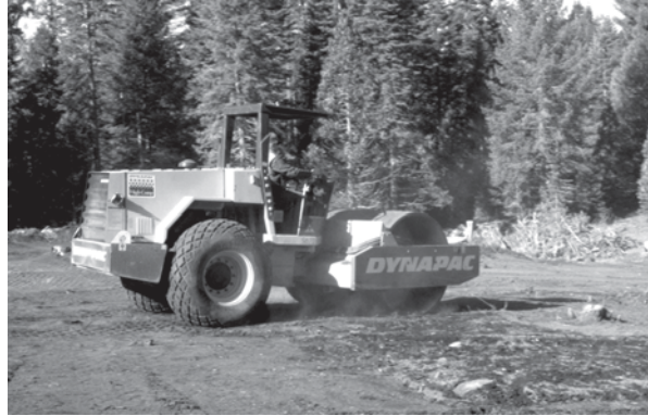
Fig. 23.9 Achieving uniform soil compaction at Challenge through perpendicular passes of a vibrating roller
