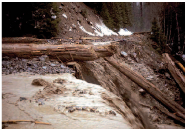
Fig. 16.9 Road in H. J. Andrews Experimental Forest rapidly eroding because of flow diversion. (Grant and Swanson 2007)
