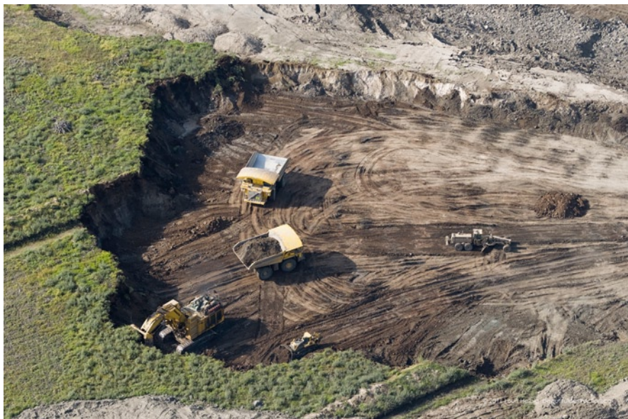
Fig. 5.4 Overburden removal for mining operations. Louis Helbig. Beautiful Destruction overburden removal B2410245
