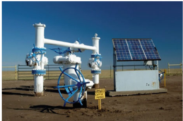
Fig. 12 Solar-electric powered pumps. (© 2012 GenPro Energy Solutions)
