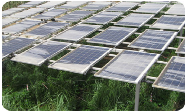
Fig. 13 Solar electric photovoltaics over TerraSave wastewater treatment system Neuschafer (2012). (© 2012 TerraSave)
