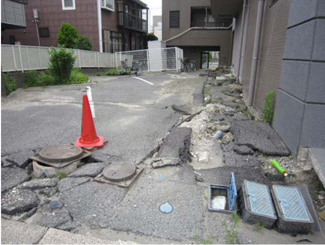
Photo 20.1 Discontinuous residence receives liquefaction damage by 2011 Tohoku earthquake in Urayasu City
