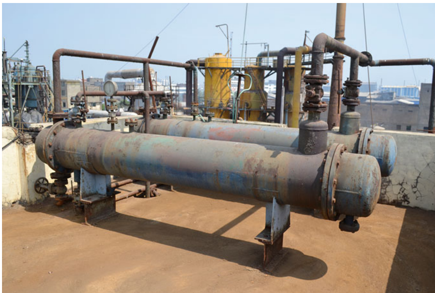
A Closeup of Liquid SO 2 Condensers at 14 M Level of M/s. Nath Industrial Chemicals Limited—VAPI, GIDC, India.
