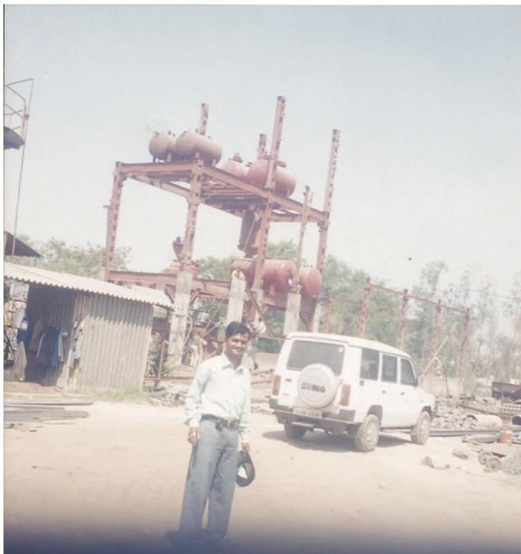
Liquid SO 2 plant installation being carried out for 15 TPD liquid SO 2 plant for M/s. Amal Rasayan Ltd in 2004-05.
