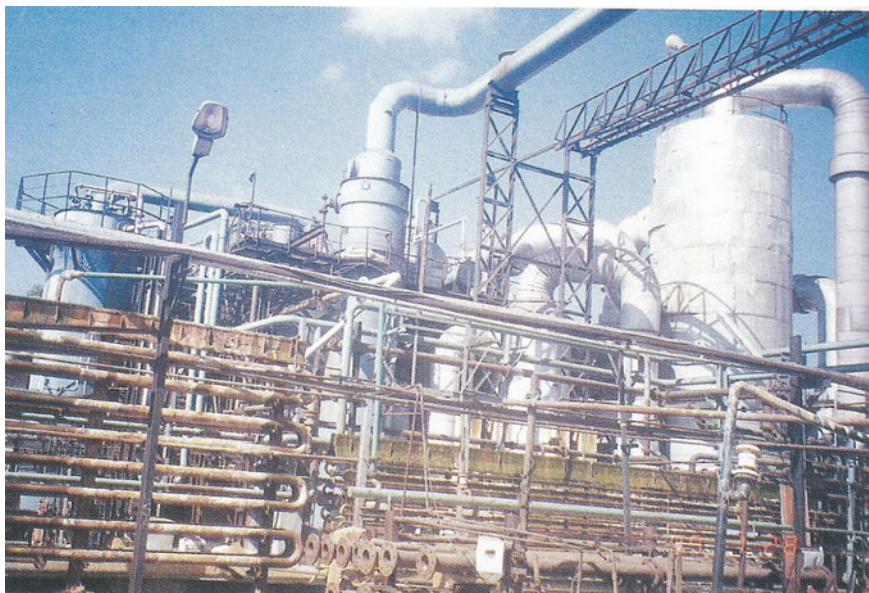
A closer look at a 180 TPD S.A. plant at Ankleshwar, Gujarat of M/s. Shree Sulphuric Acid. In the foreground one can see the Trombone Cooler for 25 % oleum.
