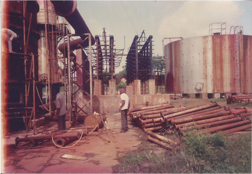
Duct from Economiser at Belagula plant of M/s. Bangur Fertiliser Chemicals in June 1992. In the foreground you can see the acid and cooler pipe with support rack and basins.
