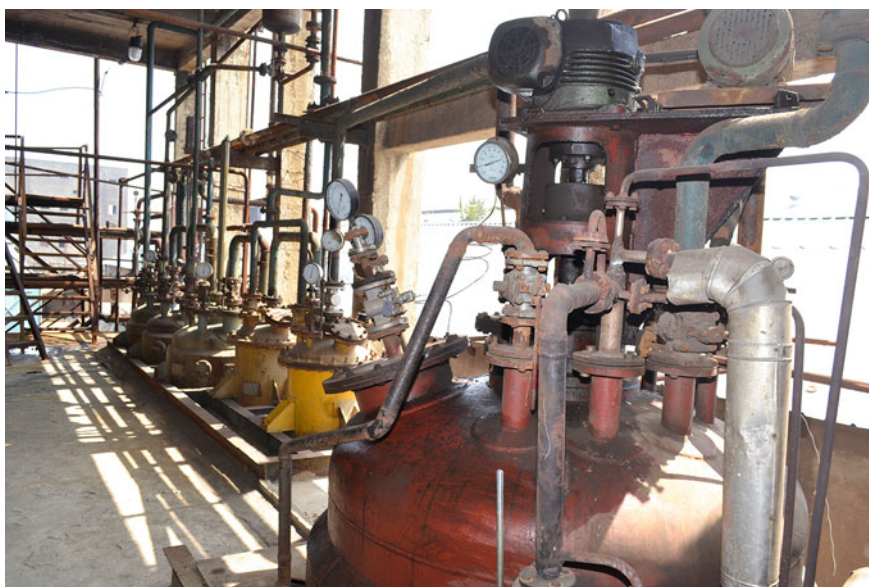
A Closeup of high pressure reactor for 20 TPD Liquid \text{SO}_2 plant of M/s. Nath Industrial Chemicals Limited—VAPI, GIDC, India.
