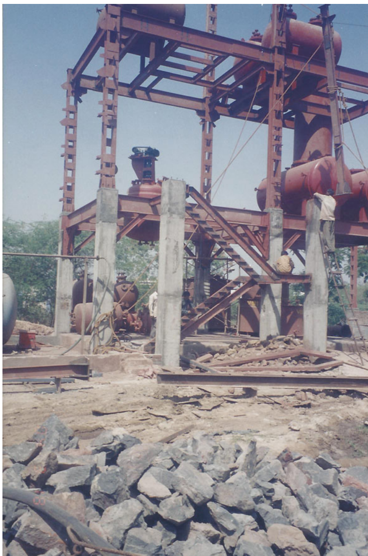
15 TPD liq SO 2 plant under construction by NEAT at M/s. Amal Rasayan Ltd at Ankleshwar, GIDC, Gujarat.
