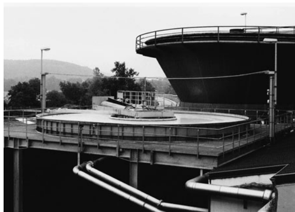
Fig. 12.4. 55 ft-diameter DAF clarifier.
