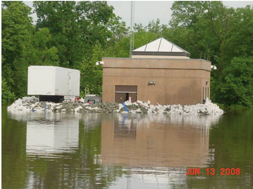
Fig. 5.5 Floodwater covering the pump house of well 4 of Cedar Rapids, Iowa during the flood of 2008. (Photo from Roy Hesemann)
