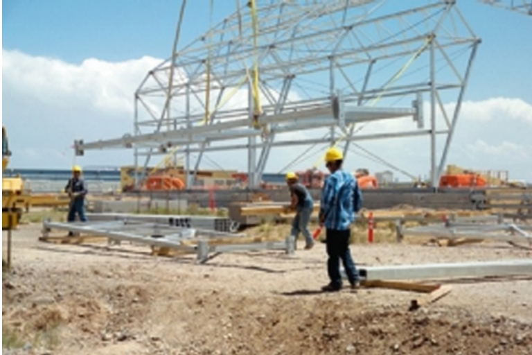
Fig. 17.2 Workers install steel structure frame for Pit 4 Retrieval Enclosure Structure at Idaho National Laboratory (DOE Photo, 2004)
