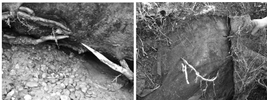
Fig. 9.6 Roots and rhizomes of Phragmites australis puncturing LDPE liner at the base and side of the reed bed
