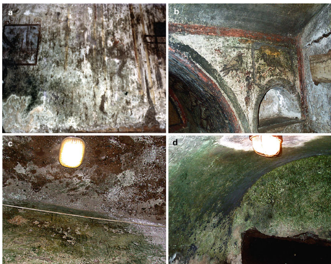
Fig. 11.5 Indoor development of phototrophic biofilms: (a) Roman frescoes at the Domus aurea and (b) wall paintings at the St. Domitilla catacombs of Rome (Italy) disfigured by the presence of thick biofilms;
