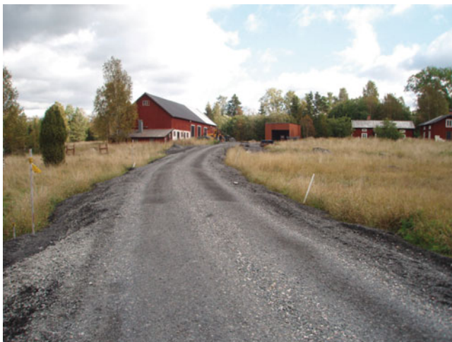
Fig. 11.1 Photograph of a stretch of the gravel road built at Tranbol using mixed wood ashes
