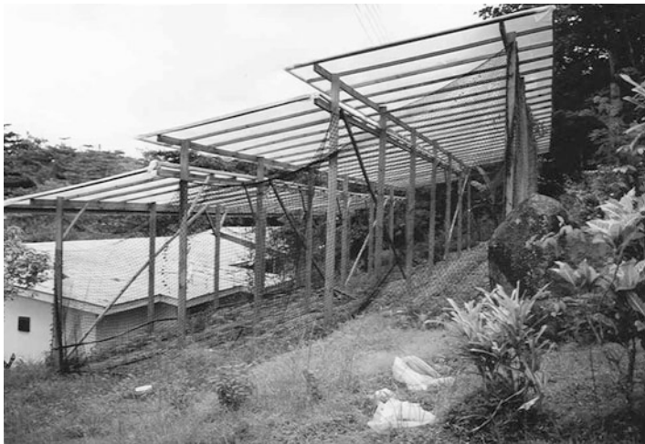
Fig. 5.77 Wooden structure for terrace shelter with nailed-on plastic film in the Seychelles
