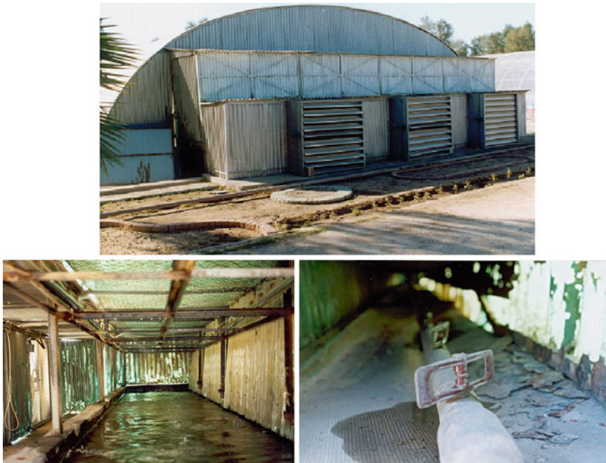
Fig. 11.36 Positive spray cooler in Kuwait 2002 (type A in Fig. 11.35), with inside view above water basin and nozzles
