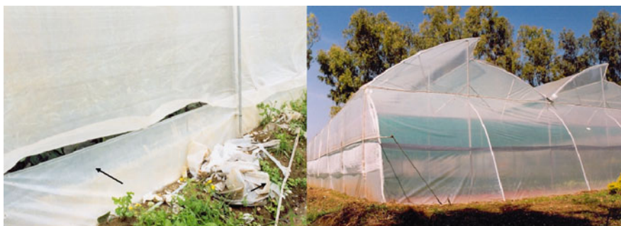
Fig. 10.15 The insect screens are not fixed tightly enough to the structure, so that leaks occur and pest insects can penetrate
