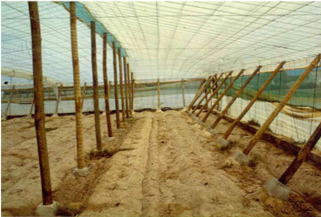
Fig. 5.68 Parral-type greenhouse in Almeria with flat roof
