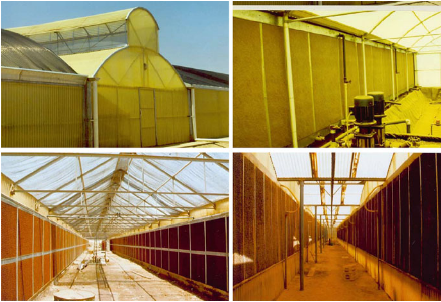
Fig. 11.19 Pads properly shaded by special roof construction or shading cloths
