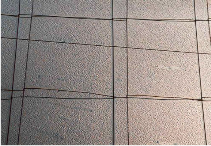
Fig. 5.69 Drop condensation on flat roofs of Parral type
