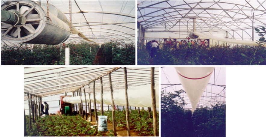
Fig. 12.7 The plastic tubes are installed too high above ground and plant level
