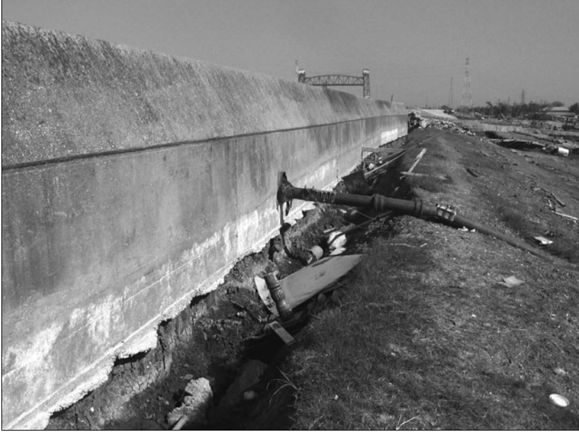
Remaining portion of Industrial Canal floodwall, October 9, 2005. Note that water had clearly come over the top of the wall, carving away the soil on the “back” side of the wall (facing the Lower Ninth Ward). Near the top of the photo is the portion of the wall that gave way catastrophically—the location from which the photo on page 101 was taken. Photograph by William Freudenburg.
