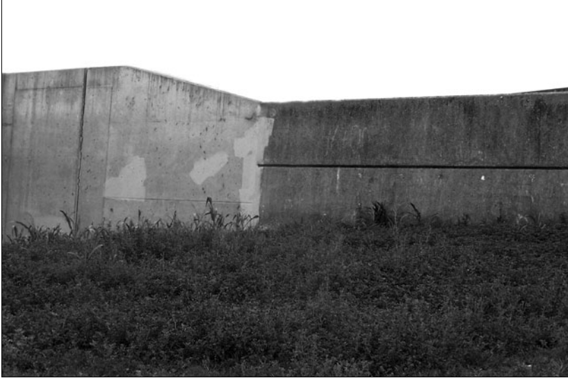
Reconstructed Industrial Canal floodwall adjoining the Lower Ninth Ward. Note differences in heights between the newer section of the wall, to the left, versus the “old” or original section/height on the right. Photograph by William Freudenburg.
