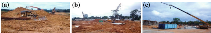
Fig. 1 Selected sites a Earthworks b Substructure (piling works) and c Superstructure works
