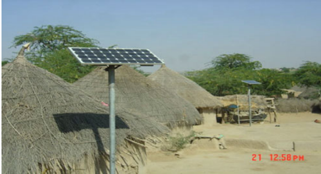
Fig. 2 A view of Solar Home System installed in Thar
