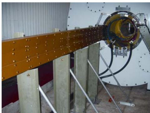
Figure 5. The gradient cables carry large direct currents through the large fringe field within the magnet room, thereby experiencing very large forces that are expected to produce eventual metal fatigue and breakage. Mechanical support severely restricts any significant movement to slow this failure onset. The gradient cables are clamped along their entire length within grooves machined into Garolite bars held in a horizontal orientation along the z -axis of the magnet from point of exit from the gradient set to the penetration panel. See attached CD for color version.
