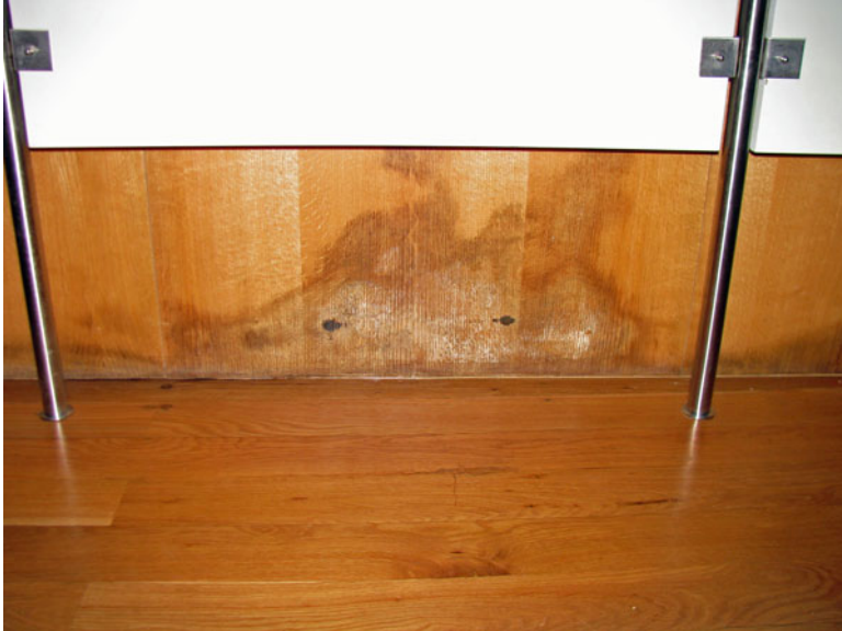
Fig. 2.6 Stains in wood materials due to water absorption
