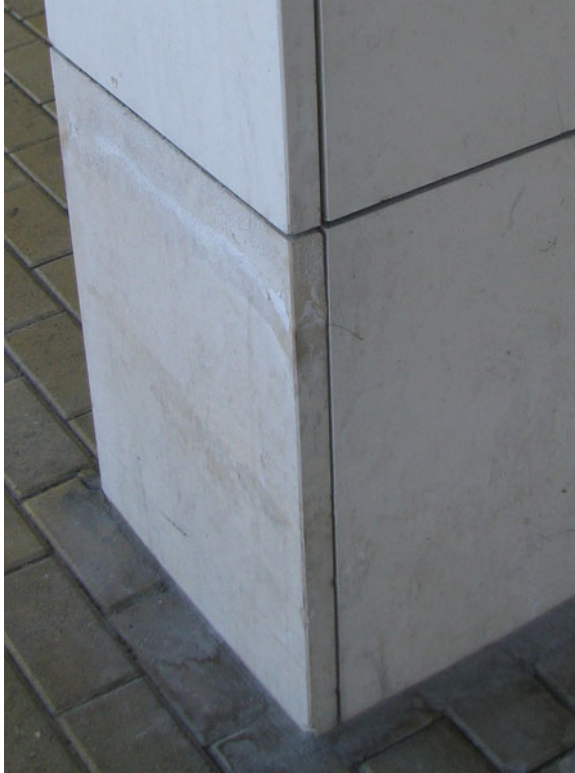
Fig. 2.9 Salt efflorescences related to capillary-rising solutions in limestones at a modern construction: note the distribution of salt efflorescences at the top of the first block, typical of water rising from the ground and where the position of the salt efflorescences results from the equilibrium between moisture feeding rate, drying rate and of solubility of the salt present at the efflorescences
