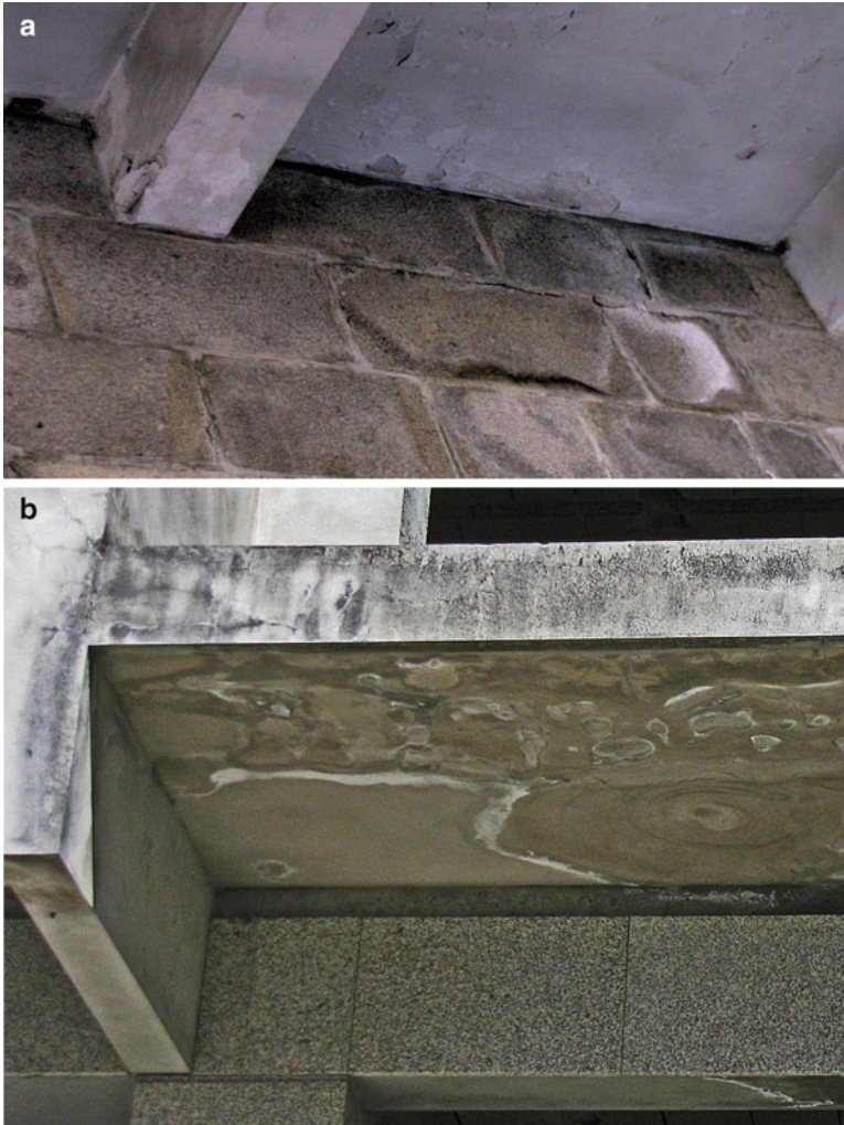
Fig. 2.8 Effects of water infiltration in historical (a) and modern constructions (b)
