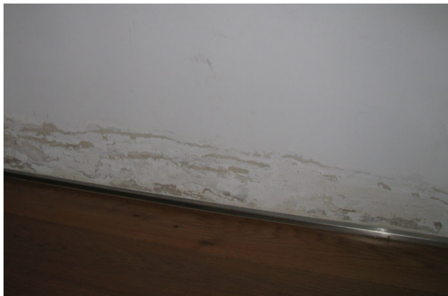
Fig. 2.5 Detachments of impermeable wall paint related to salt efflorescences
