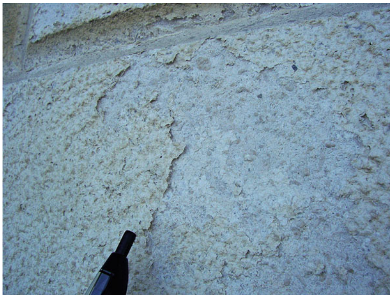
Fig. 2.3 Example of planar detachments in limestones applied in a modern construction near the sea
